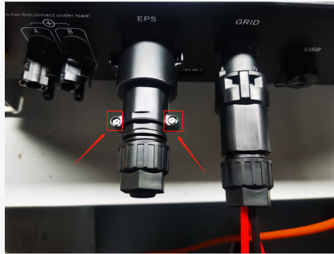
EPS port with a safety jacket
